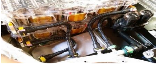
Battery Cooling System Components
